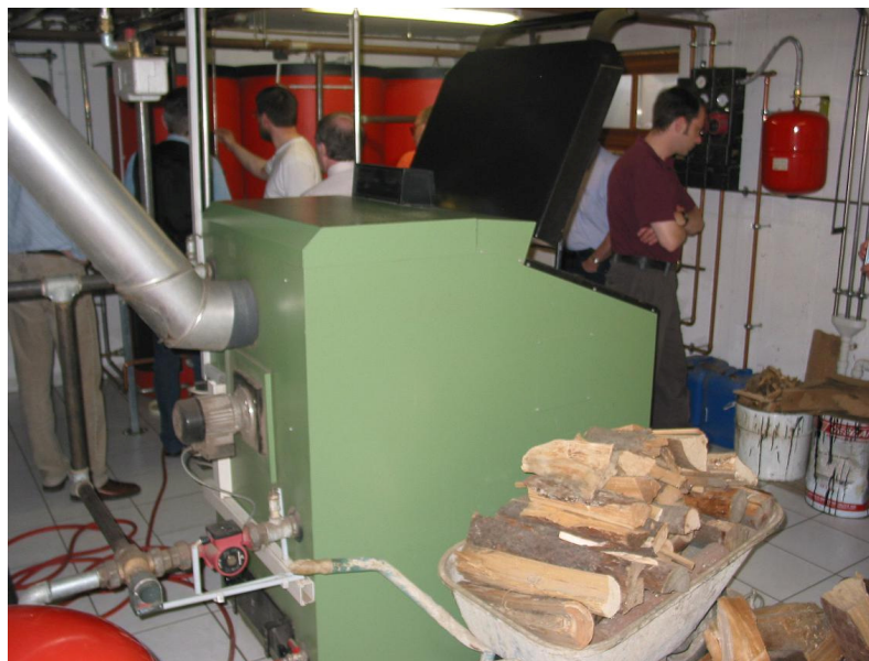
50kW log boiler with 2,800 litres of accumulator
