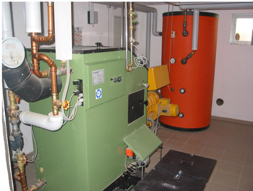
A 50 kW wood chip boiler
