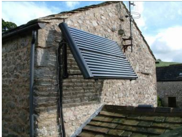
Evacuated Tube Collectors – West Barn, Malham
